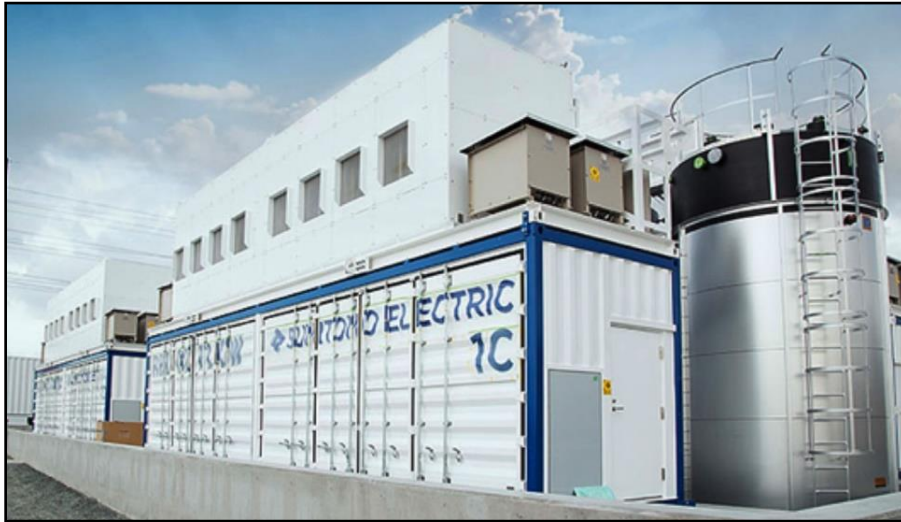
FIGURE 2.2 – Sumitomo and SDG&E's Redox Flow Battery Credit Sumitomo
