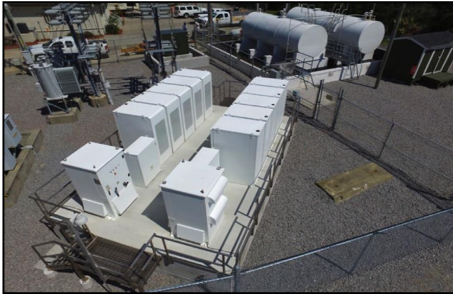
FIGURE 2.1 – Ocracoke Island li-on Battery System Courtesy of Carolina Country, NC
